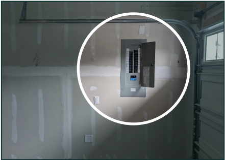
Rough-in for future electric vehicle charger & 200 AMP service
